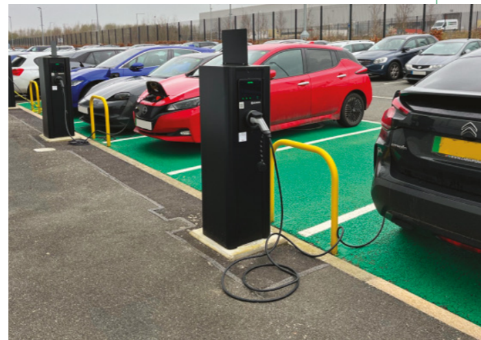
Electric vehicle charging points were installed at UK sites.
